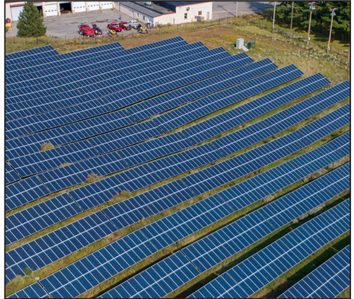
Solar array installed on town property located on Jackson Road.
