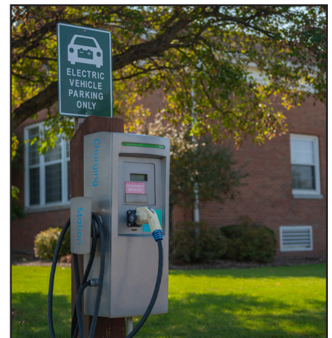
EV charging station at Penfield Town Hall campus. Penfield was the first municipality in Monroe County to install one on its property.
